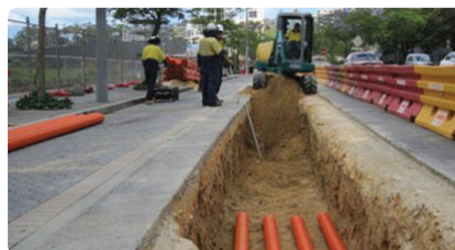
Underground Fiber Service
